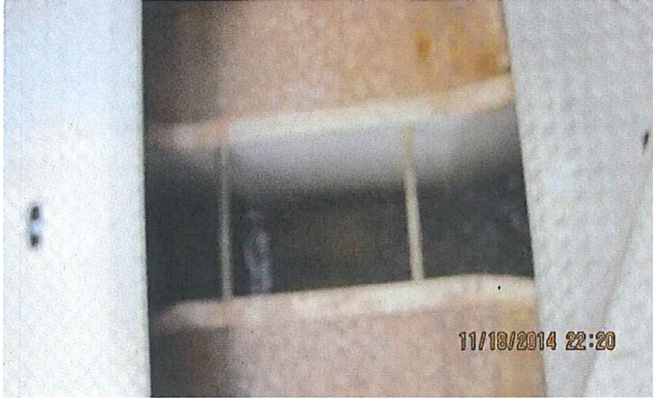
PHOTO #:05 DATE: NOVEMBER 19, 2014 TAKEN BY: CARL JONES DESCRIPTION: INFLUENT PARSHALL FLUME
