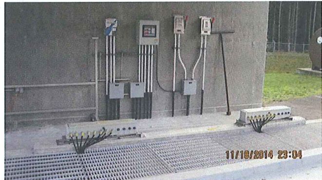
PHOTO #:13 DATE: NOVEMBER 19, 2014 TAKEN BY: CARL JONES DESCRIPTION: UV DISINFECTION CHANNEL
