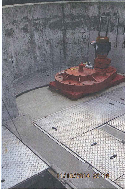
PHOTO #:02 NOVEMBER 19, 2014 TAKEN BY: CARL JONES DESCRIPTION: HEADWORKS - PISTA GRIT CHAMBER
