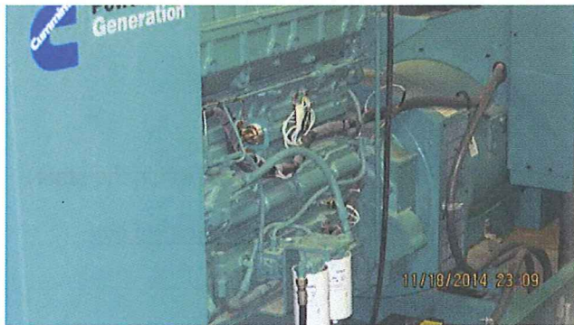
PHOTO #: 20 DATE: NOVEMBER 19, 2014 TAKEN BY: CARL JONES DESCRIPTION: BACKUP POWER GENERATOR
