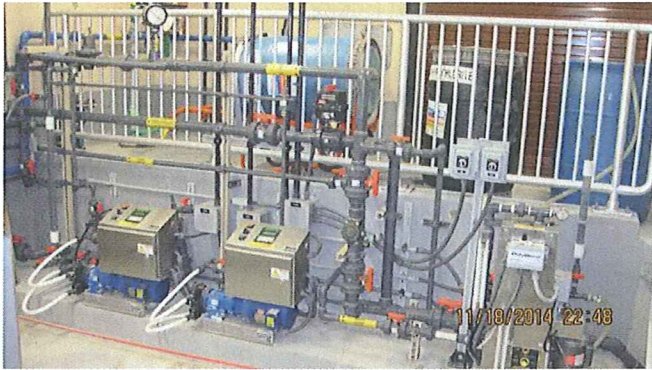
PHOTO #:18 DATE: NOVEMBER 19, 2014 TAKEN BY: CARL JONES DESCRIPTION: CHEMICAL FEED SYSTEM FOR GBT, ODOR CONTROL AND FILAMENTOUS CONTROL
