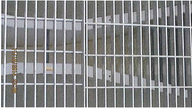
PHOTO #:14 DATE: NOVEMBER 19, 2014 TAKEN BY: CARL JONES DESCRIPTION: EFFLUENT PARSHALL FLUME
