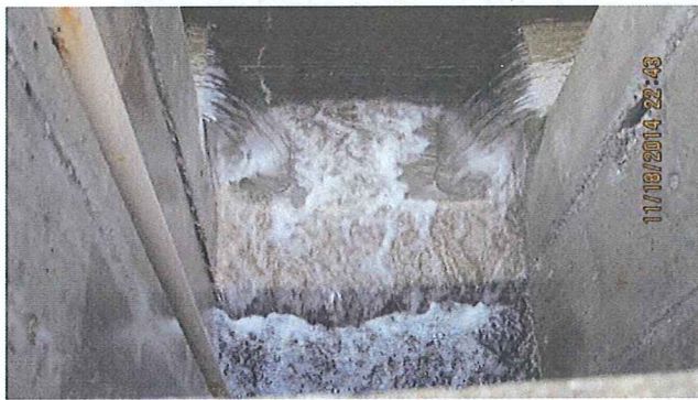
PHOTO #:12 DATE: NOVEMBER 19, 2014 TAKEN BY: CARL JONES DESCRIPTION: SECONDARY CLARIFIER EFFLUENT CHANNEL
