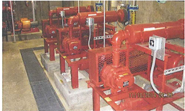
PHOTO #:08 DATE: NOVEMBER 19, 2014 TAKEN BY: CARL JONES DESCRIPTION: SINGLE-STAGE CENTRIFUGAL BLOWERS
