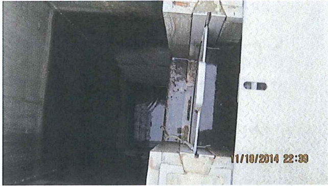
PHOTO #:10 DATE: NOVEMBER 19, 2014 TAKEN BY: CARL JONES DESCRIPTION: CLARIFIER INFLUENT SPLITTER BOX AND FLOW GATE
