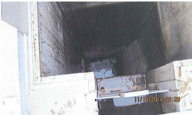
PHOTO #:09 DATE: NOVEMBER 19, 2014 TAKEN BY: CARL JONES DESCRIPTION: SECONDARY CLARIFIER INFLUENT SPLITTER BOX AND WET WELL
