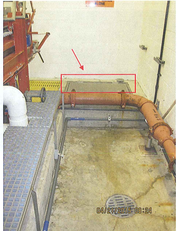
PHOTO # 28 DATE: 04/21/2015 TAKEN BY: LAZARO ELEUTERIO DESCRIPTION: TWAS STORAGE TANK (UNDERGROUND)
