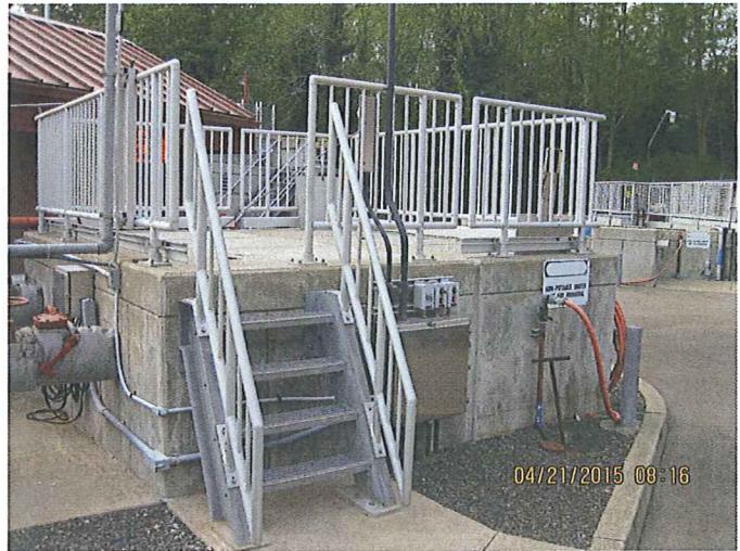
PHOTO # 16 DATE: 04/21/2015 TAKEN BY: LAZARO ELEUTERIO DESCRIPTION: AERATION BASINS FLOW SPLITTER BOX (UPSTREAM OF SECONDARY CLARIFIERS)
