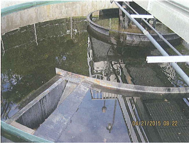
PHOTO # 19 DATE: 04/21/2015 TAKEN BY: LAZARO ELEUTERIO DESCRIPTION: SECONDARY CLARIFIER # 2
