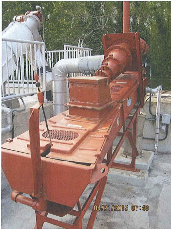
PHOTO # 5 DATE: 04/21/2015 TAKEN BY: LAZARO ELEUTERIO DESCRIPTION: GRIT CYCLONE AND CLASSIFIER
