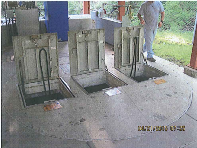
PHOTO # 1 DATE: 04/21/2015 TAKEN BY: LAZARO ELEUTERIO DESCRIPTION: INFLUENT WET WELL (INFLUENT PUMP STATION)
