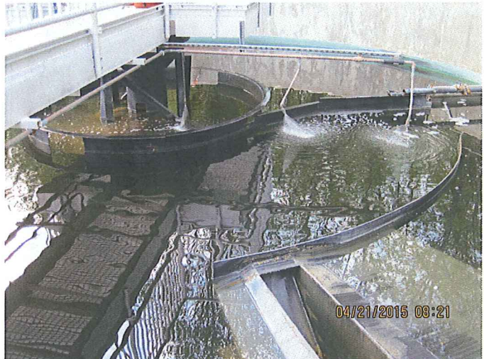
PHOTO # 18 DATE: 04/21/2015 TAKEN BY: LAZARO ELEUTERIO DESCRIPTION: SECONDARY CLARIFIER # 1
