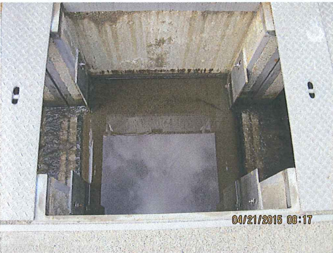
PHOTO # 17 DATE: 04/21/2015 TAKEN BY: LAZARO ELEUTERIO DESCRIPTION: AERATION BASINS FLOW SPLITTER BOX (DETAIL)
