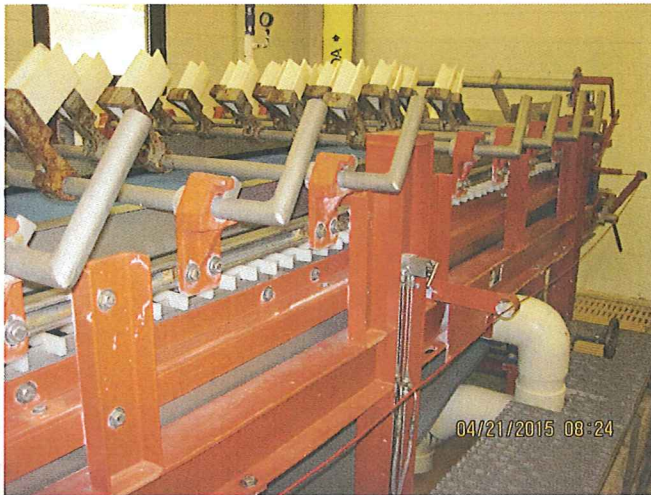
PHOTO # 27 DATE: 04/21/2015 TAKEN BY: LAZARO ELEUTERIO DESCRIPTION: GRAVITY BELT THICKENER (GBT)
