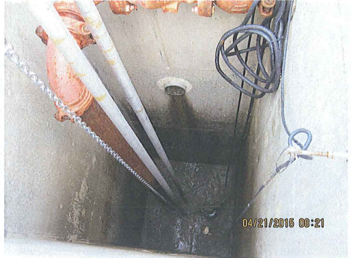
PHOTO # 20 DATE: 04/21/2015 TAKEN BY: LAZARO ELEUTERIO DESCRIPTION: SECONDARY CLARIFIERS SCUM BOX
