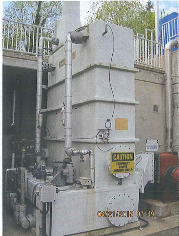
PHOTO # 8 DATE: 04/21/2015 TAKEN BY: LAZARO ELEUTERIO DESCRIPTION: ODOR SCRUBBER SYSTEM
