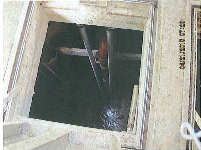
PHOTO # 2 DATE: 04/21/2015 TAKEN BY: LAZARO ELEUTERIO DESCRIPTION: INFLUENT WET WELL (DETAIL)
