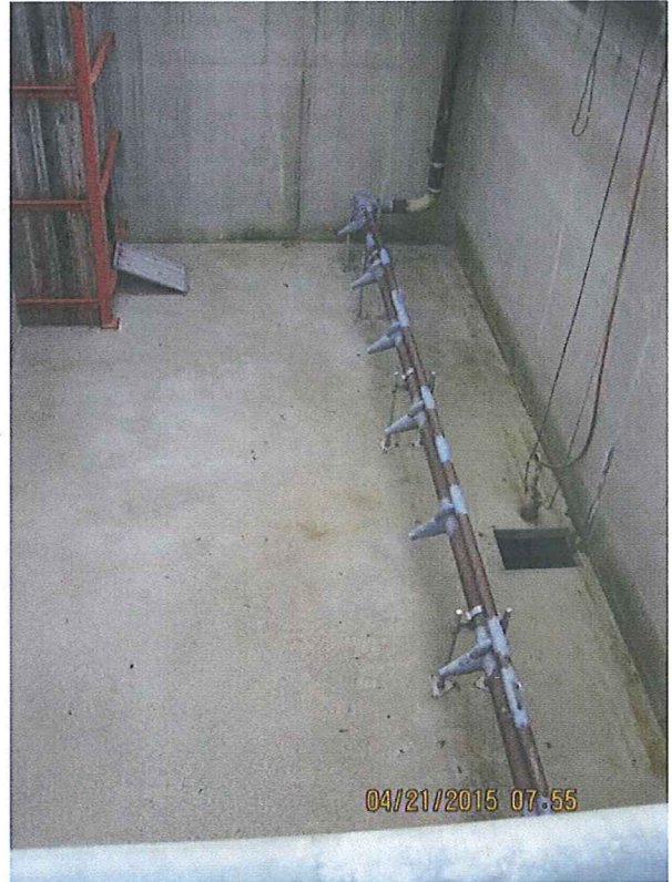
PHOTO # 12 DATE: 04/21/2015 TAKEN BY: LAZARO ELEUTERIO DESCRIPTION: AERATION BASIN # 2
