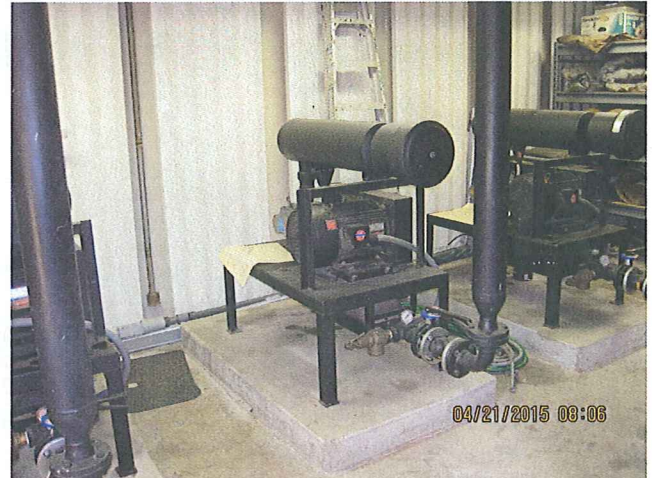
PHOTO # 14 DATE: 04/21/2015 TAKEN BY: LAZARO ELEUTERIO DESCRIPTION: AERATION BASINS' BLOWERS
