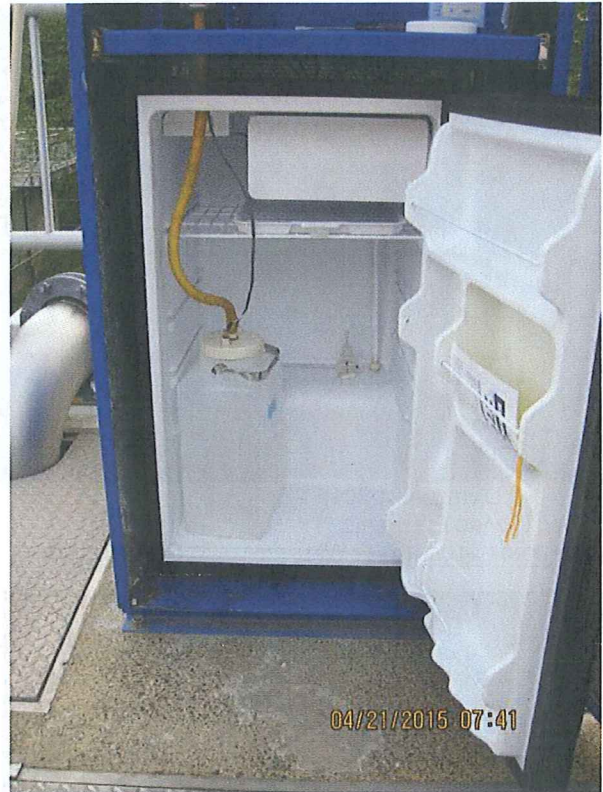
PHOTO # 6 DATE: 04/21/2015 TAKEN BY: LAZARO ELEUTERIO DESCRIPTION: INFLUENT COMPOSITE SAMPLER
