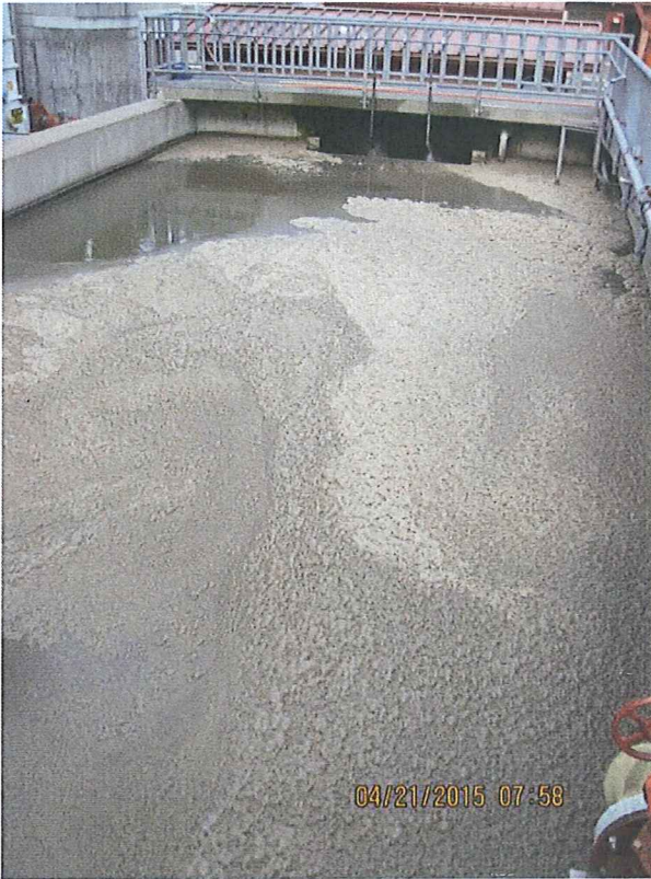
PHOTO # 11 DATE: 04/21/2015 TAKEN BY: LAZARO ELEUTERIO DESCRIPTION: AERATION BASIN # 1
