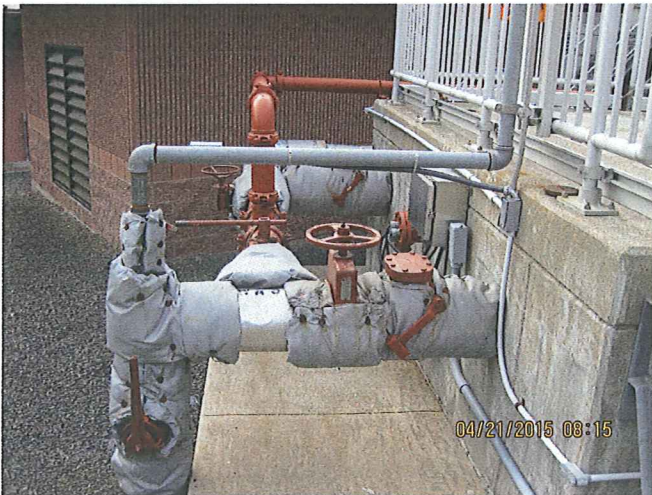
PHOTO # 15 DATE: 04/21/2015 TAKEN BY: LAZARO ELEUTERIO DESCRIPTION: RETURN ACTIVATED SLUDGE (RAS) STATION
