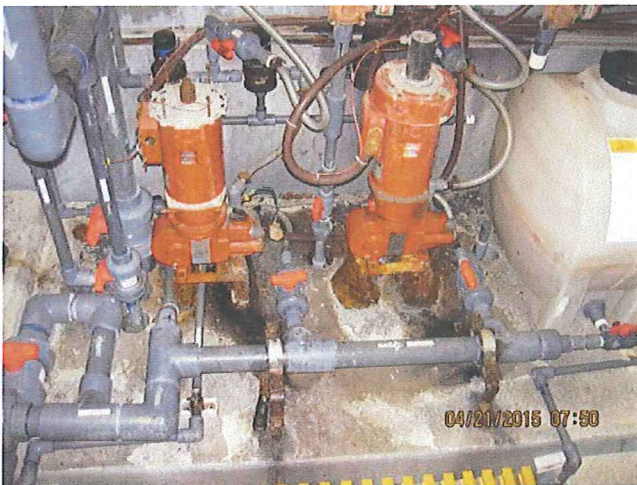
PHOTO # 9 DATE: 04/21/2015 TAKEN BY: LAZARO ELEUTERIO DESCRIPTION: ODOR SCRUBBER CHEMICAL FEED SYSTEM
