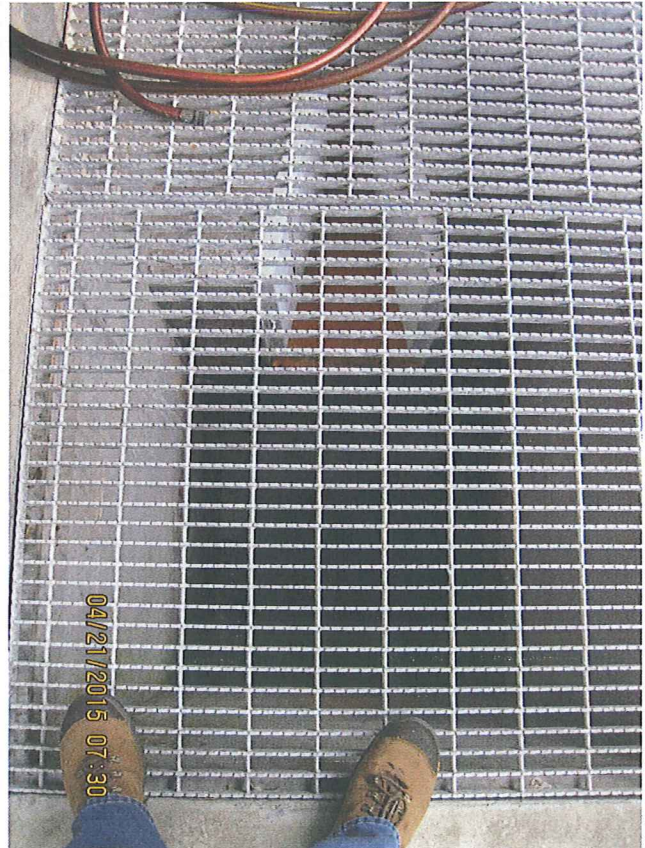
PHOTO # 22 DATE: 04/21/2015 TAKEN BY: LAZARO ELEUTERIO DESCRIPTION: EFFLUENT PARSHALL FUME
