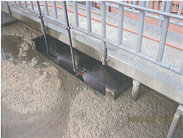
PHOTO # 13 DATE: 04/21/2015 TAKEN BY: LAZARO ELEUTERIO DESCRIPTION: WATER SPRAY FOR SCUM CONTROL
