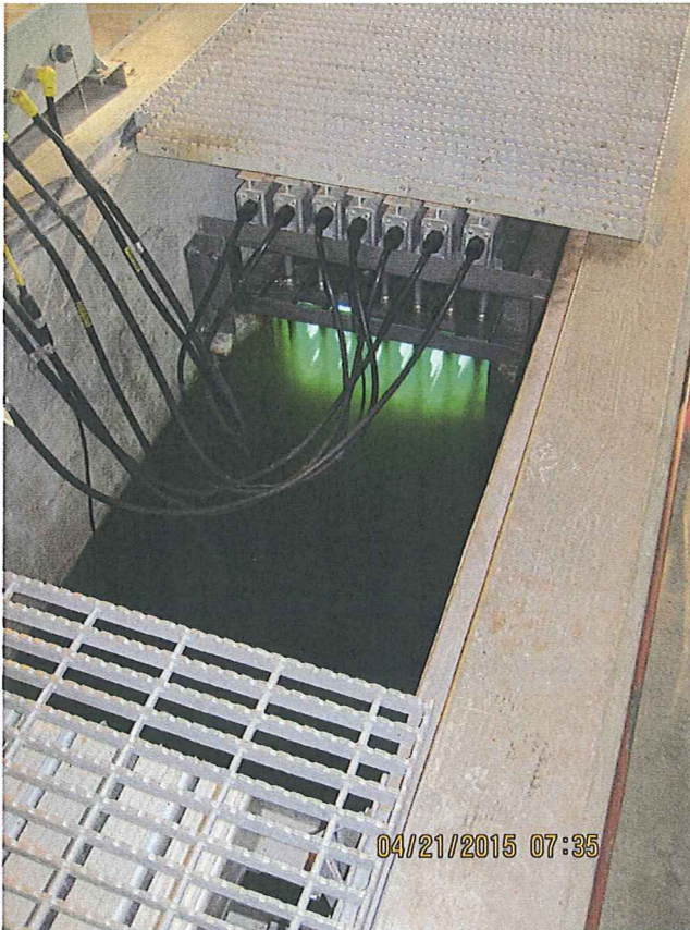
PHOTO # 21 DATE: 04/21/2015 TAKEN BY: LAZARO ELEUTERIO DESCRIPTION: UV DISINFECTION SYSTEM
