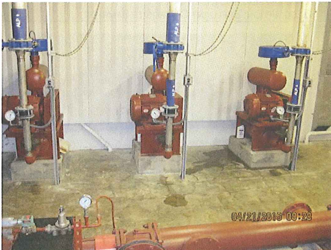
PHOTO # 29 DATE: 04/21/2015 TAKEN BY: LAZARO ELEUTERIO DESCRIPTION: WAS AND TWAS STORAGE TANKS' BLOWERS
