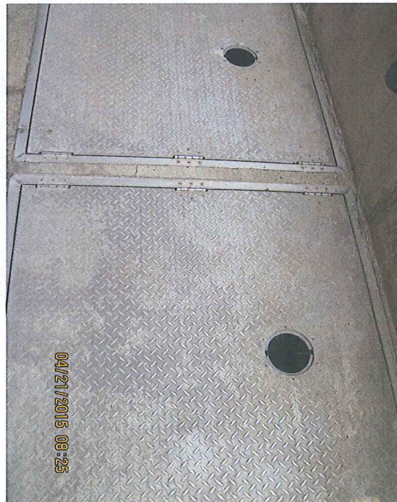
PHOTO # 26 DATE: 04/21/2015 TAKEN BY: LAZARO ELEUTERIO DESCRIPTION: WAS STORAGE TANKS
